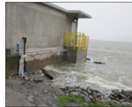
King tides at the furthest land accessible point on EBMUD's Bay outfall, a structure not usually surrounded by water. Photo courtesy EBMUD.
