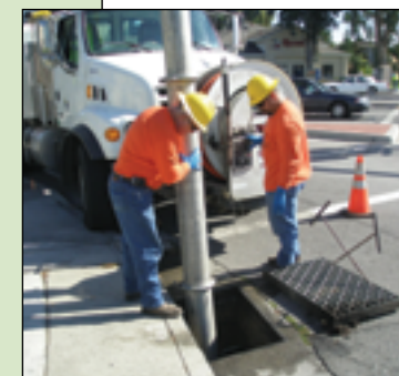
Workers vacuum storm drain in Sunnyvale to remove contaminated sediment. Photo courtesy Santa Clara Valley Stormwater Program.
